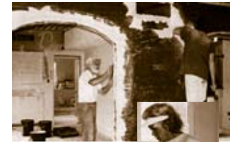
The Kreitzer family working on the walls inside the new WAS-H building.
